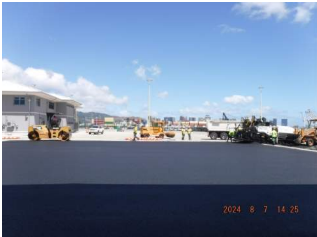
PCCP: PASHA maintenance block out - HMA paving completed at 1430 hours, crew cleaning up.
