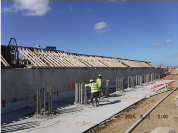
Pier 42: KIWC civil crew continued to chip the concrete over pour over the 36-inch CIDH piers
