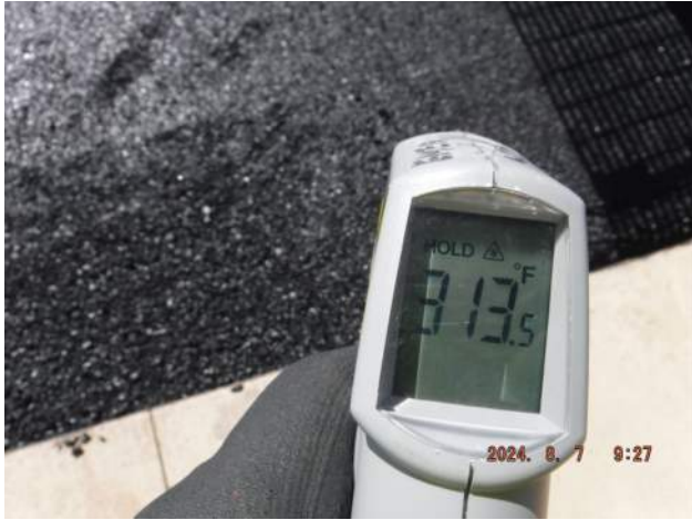
PCCP: PASHA maintenance block out -Fron of the paver the temperature was measured at 313.0 deg F.
