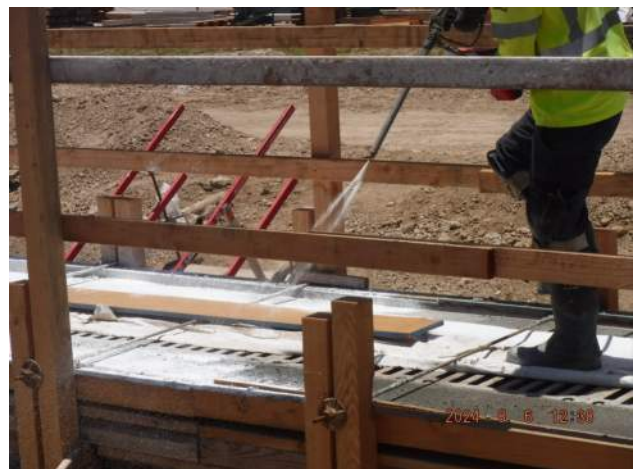
Pier 41: KIWC mason crew sprayed the concrete waxy compound for concrete curing
