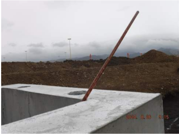
Pier 42: PECL installed the electrical electric grounding rod in PBC9 and PBE9
