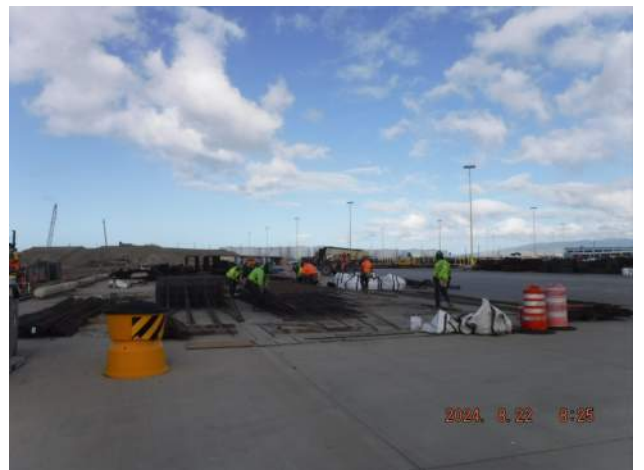
PCCP: Lay down area - HRSPI crew pre-fabricating the steel rebar cage for the trench drain (TD2)
