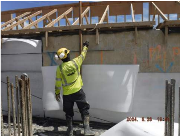
Pier 42: KIWC mason crew continued to install the expansion board of the WSCR
