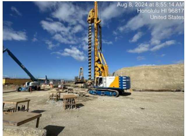
PF predrilling near the installed 48" CIDH shafts in the junction structure SOE area
