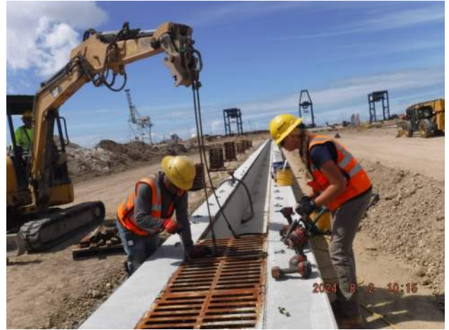
Pier 41: KIWC carpentry crew (Philip's) installed the frames and grates of P1 to P3 of trench drain 3
