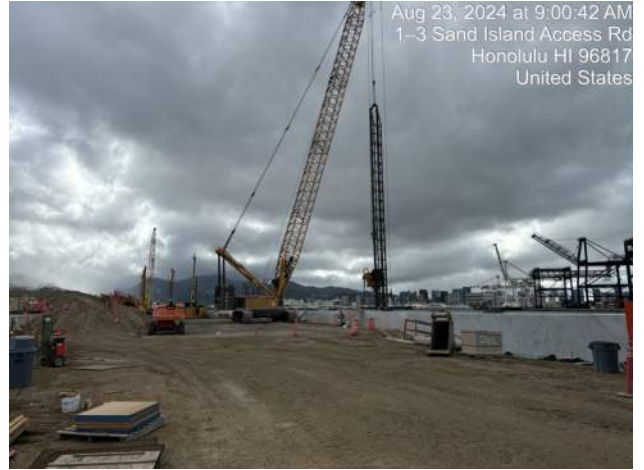
KIWC prepping to probe the outside of the cap beam on Pier 43
