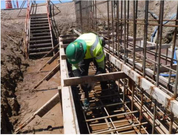
Pier 40F: HRSPI crew cut the end of the rebar to accommodate 3-inch clearance per MN structural observations Photo #1
