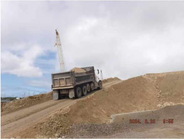
Pier 41: KIWC civil crew hauled the processed dredged material into Snug Harbor surcharge fill
