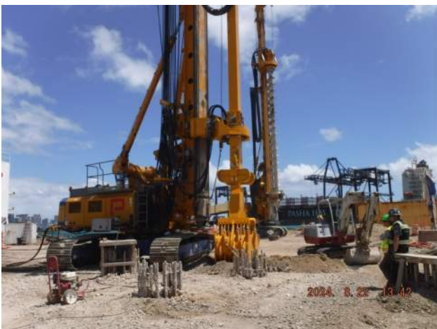
Pier 42: PFoundation started to drill the area surrounding the existing 48-inch CIDH pier
