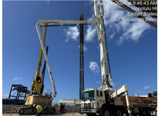
View of typical rebar cage for CIDH while hole is being cleaned out by drill rig
