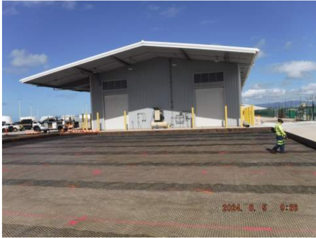
PCCP: PASHA maintenance blockout- Road Builders crew sprayed SS-1 asphalt emulsion on the sides of the PCCP
