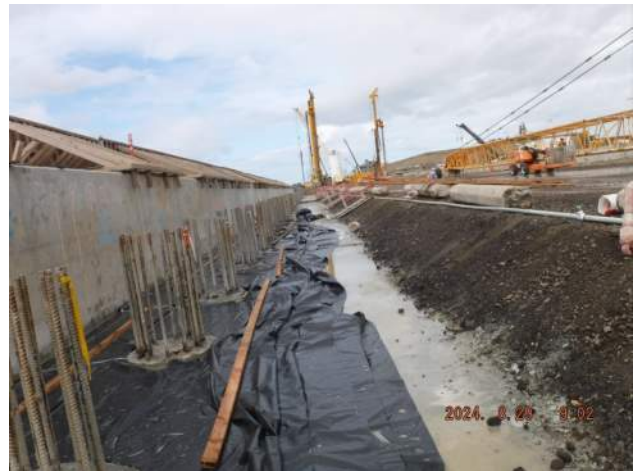
Pier 42: KIWC carpentry crew (Philip's) installed the PVC polyvinyl sheet bond breaker from STA 16+00 to STA 15+70
