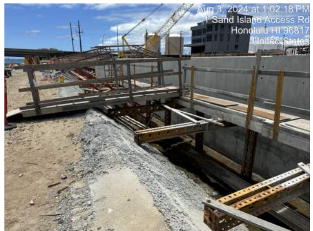
KIWC performing the dry finish for the waterside of the cap beam on P22
