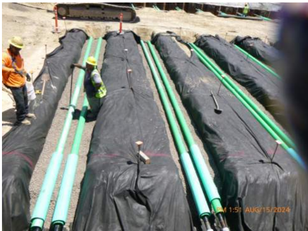
KIWC setting tie rods in the tie rod trenches between the LSCRB and the combi wall.
