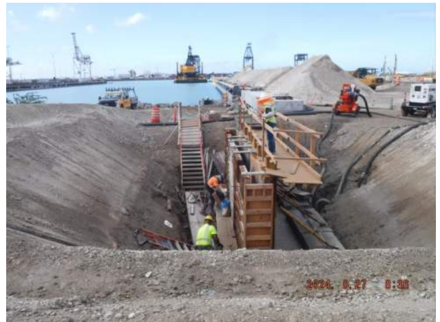
Pier 40F: KIWC carpentry crew continued to finalized the installation of the upper headwall forms
