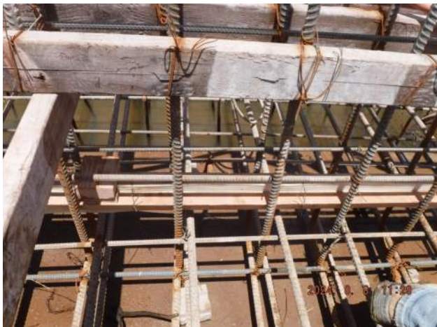
Pier 40F: KIWC carpentry crew continued to install the Sika 701 water stop in the keyway of the storm drain headwall
