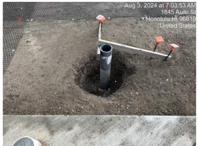
KIWC prepped to pour CLSM around the sewer cleanout pipe in the Pasha Maintenance Building blockout
