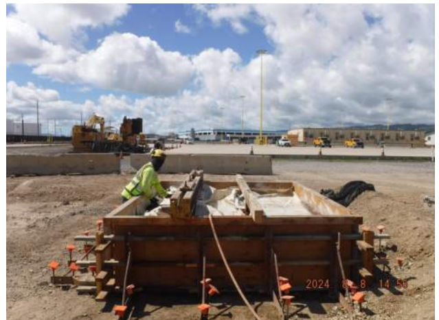
Pier 43: KIWC mason crew applied concrete curing compound for the water manhole WL-1 concrete pour
