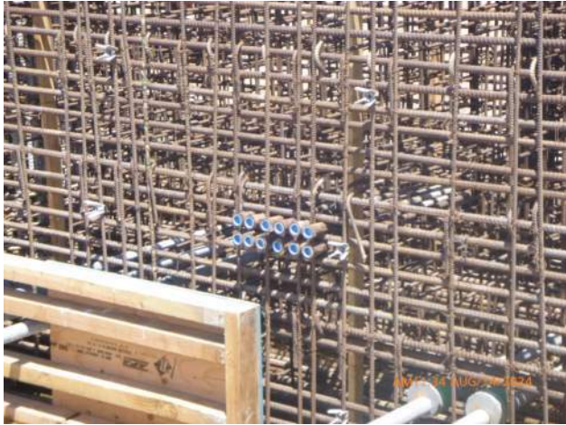
View of form savers for Tie beam dowels embedded in LSCRB pour #7.
