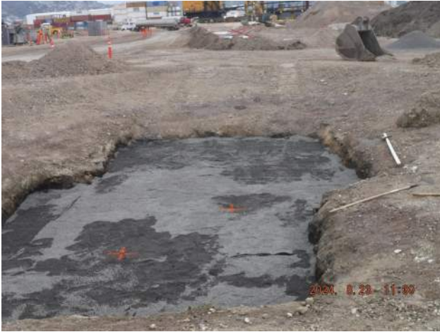
Pier 42: PECL crew grading and leveling the S4C sand for installation of the manhole bases
