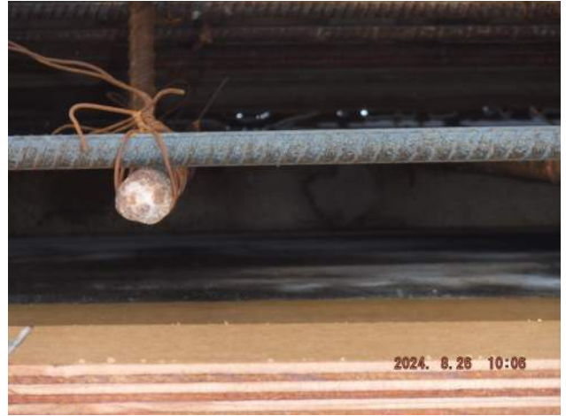
Pier 40F: Pre-pour headwall inspection found one dobie block top of the footing foundation
