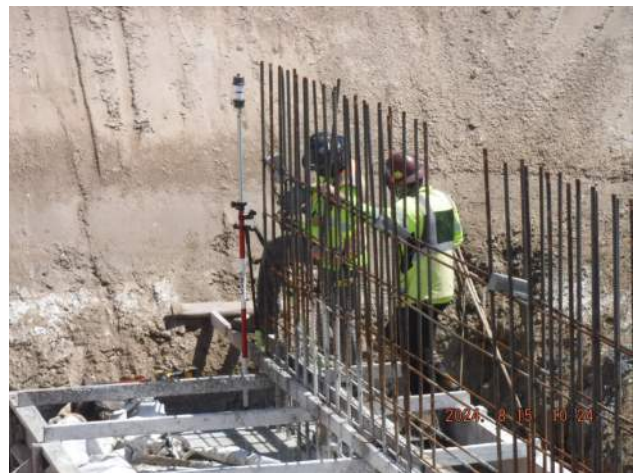
Pier 40F: HL crew surveyed the top elevation of the footing foundation of the storm drain head wall
