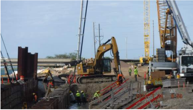
Pier 43: KIWC carpentry crew (Philip's crew) started to place the concrete mixed for the mud mat for pour P16 of the combi wall
