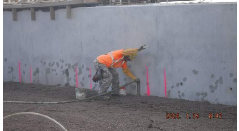
Pier 42: KIWC mason crew continued to grout the form tie holes for P3 and P4 of the CWCB
