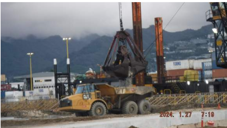
Pier 41: Loading dredged material into the bed of the CAT 730 rock truck
