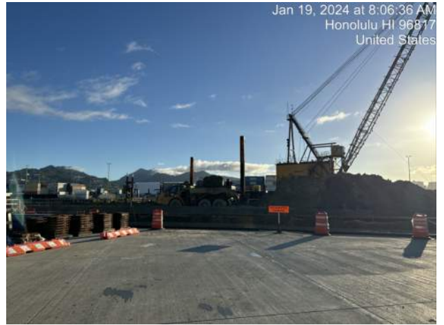
KIWC dredge support crew using the CAT 950M loader and CAT 730 dump trucks to haul material to the Snug Harbor surcharge area
