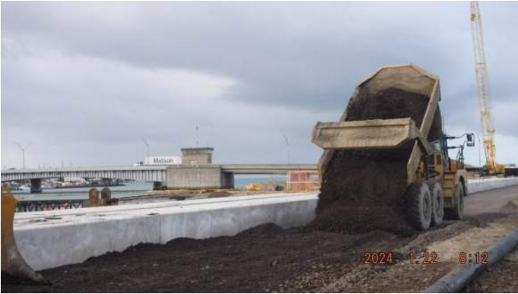
Pier 43: KIWC civil crew continued to place minus (-) 3" aggregate of the LSCRB from P2 to P6
