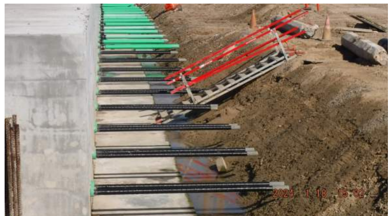
Pier 43: KIWC civil crew (Sanu's crew) taped the exposed tie rods and installed the PVC sleeves for Pour #P7
