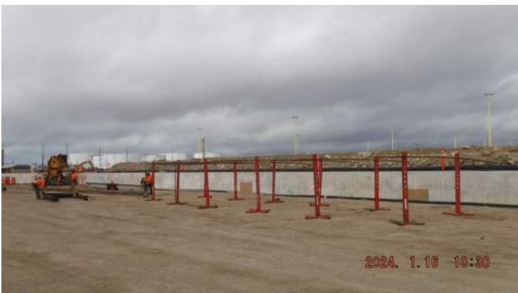
Pier 42: HRSPI crew continued to fabricate the rebar cage for Pours 14 and 15 of the CWCB
