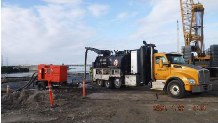
Pier 43: KIWC civil crew used the vacuum truck to suck out the muck inside the king pile annulus to -5' elevation
