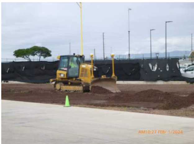
KIWC grading the pavement blockouts on the north side of the jobsite.
