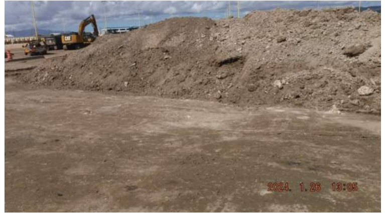
Snug Harbor: Compacted the dredge material over Grids 8, 9, and 10 of Snug at approximate elevation +10'
