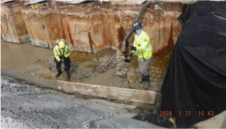
Pier 43: Between pours P22 and P23 - KIWC carpentry crew installed the steel forms for the mud mat pour
