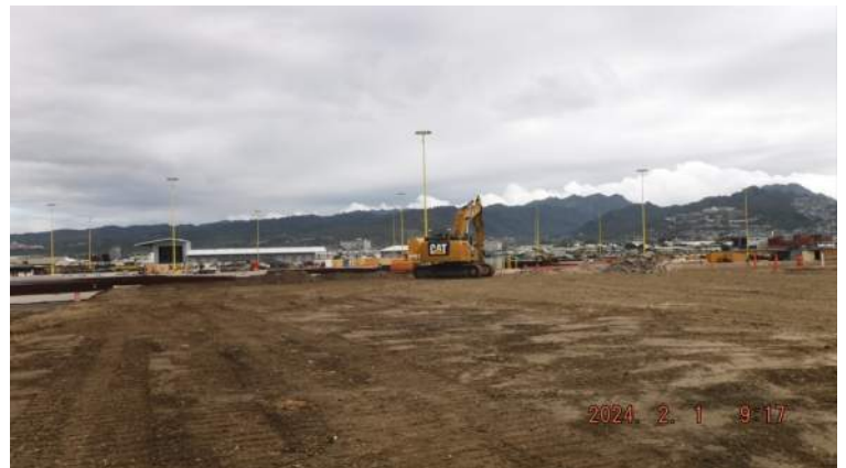
Snug Harbor: KIWC civil crew (Brent's) continued to fill the surcharge to +15 elev.
