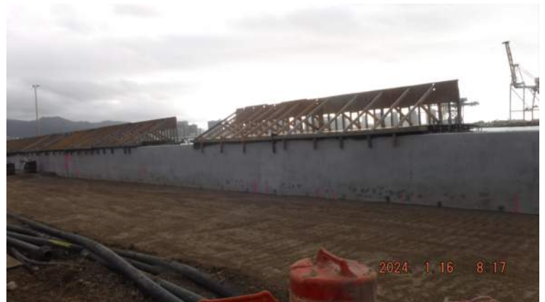
Pier 42: KIWC mason crew continued to patch the honeycombs on the wall of the CWCB of P2 to P4
