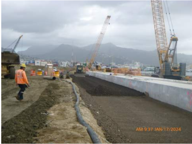
KIWC spreading an 8" loose lift of base course on the landside of the LSCRB.
