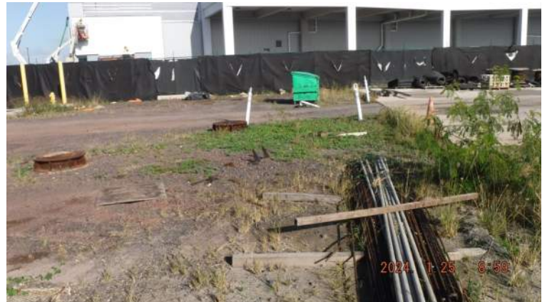
PCCP: KIWC carpentry crew used the Hyster forklift to clear off construction equipment and materials of the block out
