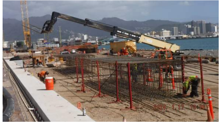
Pier 42: Laydown area (Across P14/15) HRSPI crew continued to fabricate the rebar cage of Pours P14/15 of the CWCB
