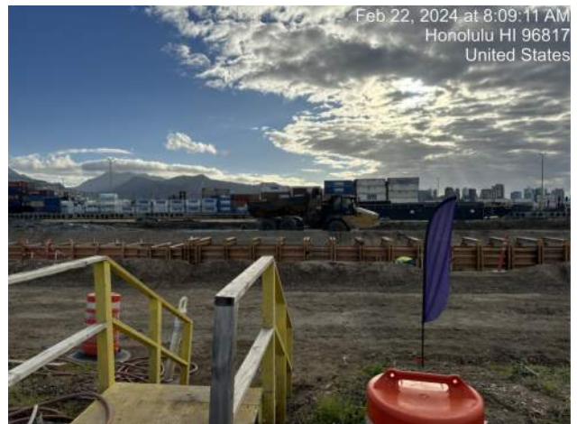
KIWC continued in-water dredging and placing material into CAT 730 dump trucks to be stockpiled on Pier 41
