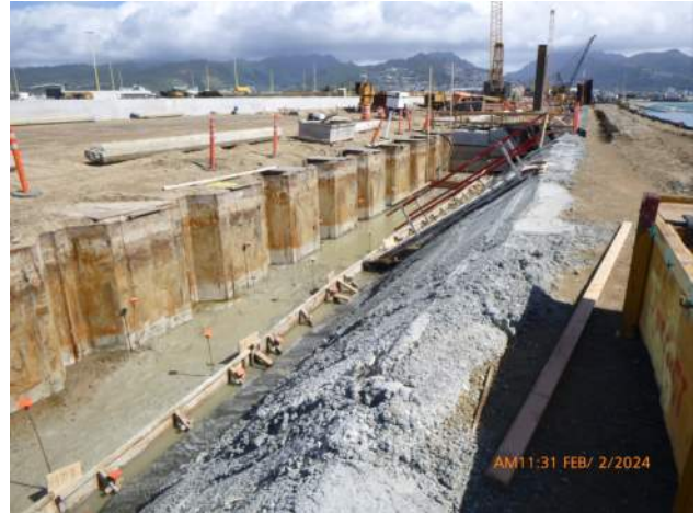
KIWC setting forms for the mud mat on the waterside of the Pier 43 combi wall.
