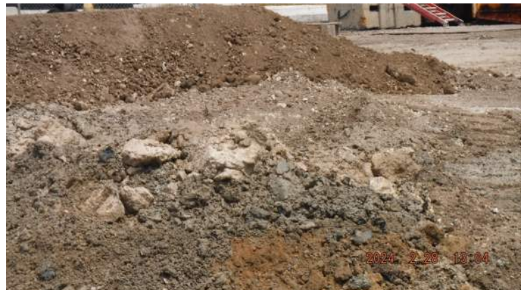
Pier 41: PO Deadman extension - Excavation spoils of coral rock and sand for the installation of the tie rods
