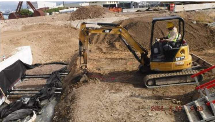
Pier 41: KIWC civil crew used the CAT 304 mini excavator to initially excavate the subgrade near the tie rods at the PO Deadman extension
