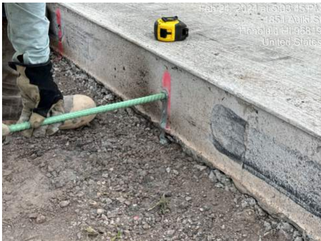
KIWC pushing the #5 rebar dowel into the drilled hole and epoxy seeping out around the dowel
