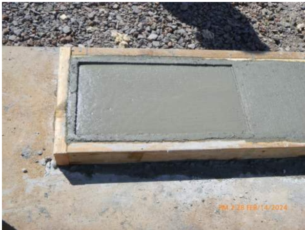
KIWC testing stamp for drain stencil.
