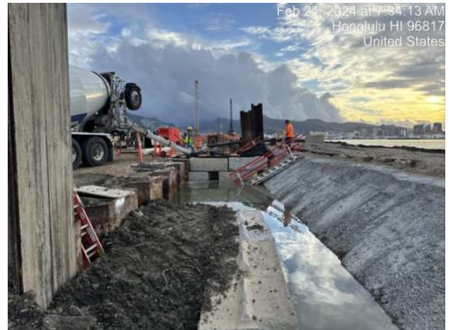
KIWC placing CLSM to create a bulkhead east and west of the SP-74 area to prevent water infiltration into the capping beam excavation after the piles are removed
