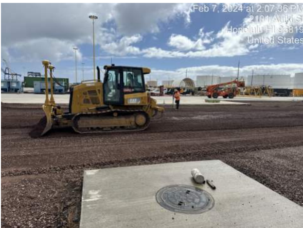
KIWC continued grading the blockout on the north end of the site
