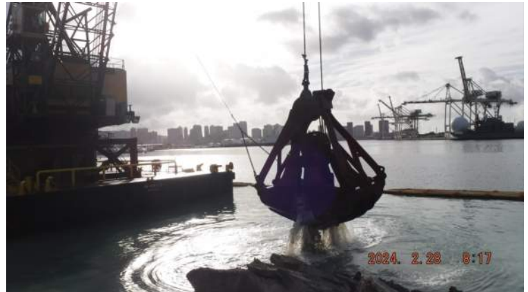
Pier 42: KIWC DB Seattle continued in water dredging across P1 of the CWCB
