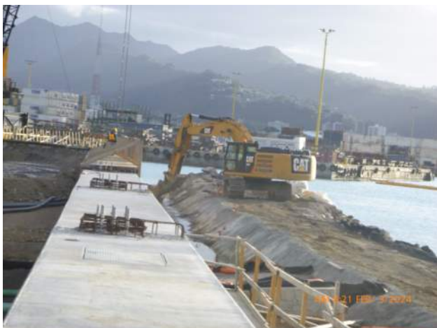
KIWC breaking up excess concrete along the wall of the capping beam excavation.
