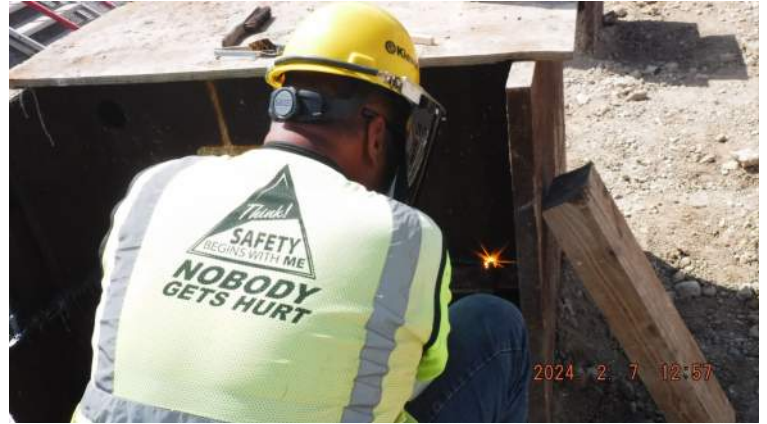
Pier 43: STA 1+69 to STA 2+60 - KIWC Bridge _Marine crew continued to cut the top of the combi wall for final top elevation
