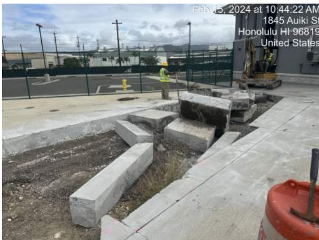
KIWC demolishing the sawcut PCC at the blockout south of the PASHA maintenance building
