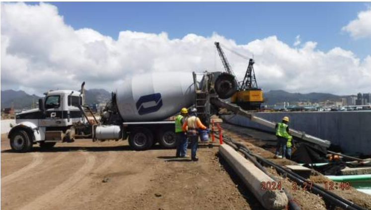
Pier 42: KIWC civil crew (Micah's crew) placed CLSM material for the water cut off wall of P6 on the land side of the CWCB
