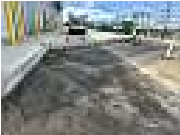
KIWC placing geogrid for the PCCP blackout between the Pasha maintenance area and parking lot
