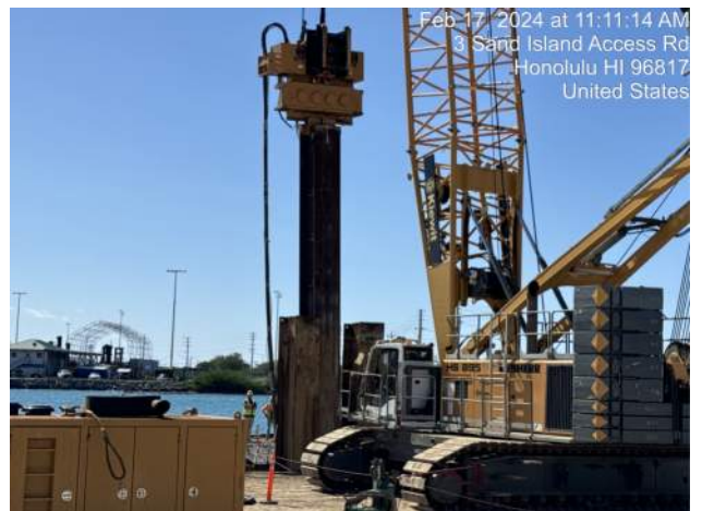
KIWC drove the follower king pile on the east end of location SP-74 on Pier 43
