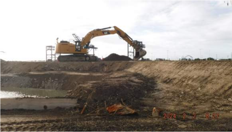
Snug Harbor: KIWC civil crew placing the first lift grids 19 and 33 of Snug
