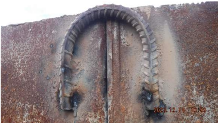
2023.12.18 10:59 Pier 42: KIWC Bridge and Marine crew continued to weld the "U" bar between the king and sheet piles interlocks
