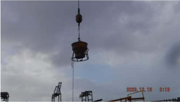
Pier 42: KIWC carpentry crew poured concrete for the reaction block on the corners of Pier 41/42
