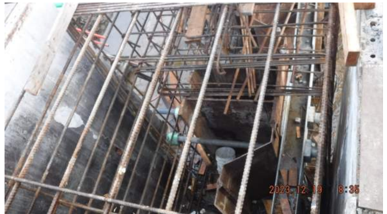
2023.12.19 8:35 Pier 42: KIWC Carpentry crew (Pihilip's crew) continued to strip the bulkhead of P11 of the CWCB
