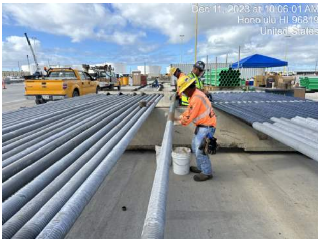
KIWC installing the double layer tape wrap system for the tie rods on the PCC
