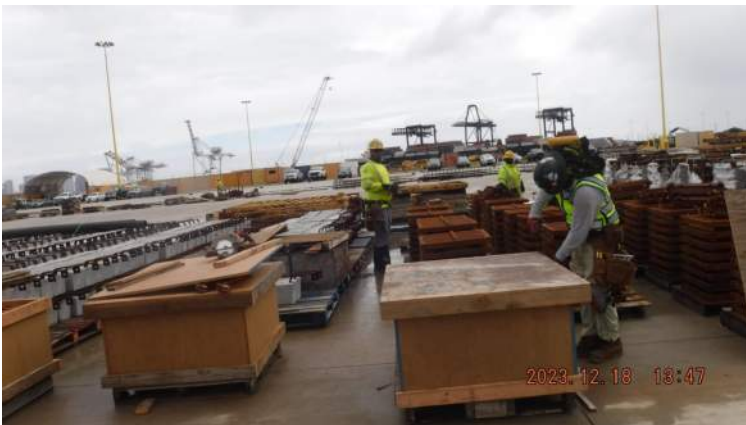
2023.12.18 18:47 PCCP: KIWC carpentry crew continued to separate the grating from the support braces by unbolting the nuts and bolts
