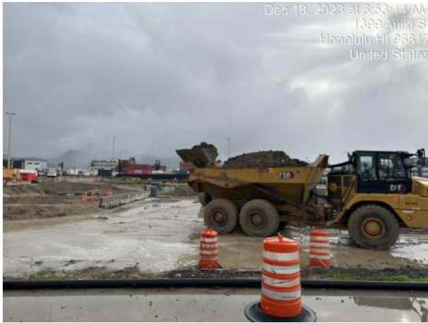
Dec 16, 2023 at 8:53:14 AM 1399 Aiea St Honolulu HI 96817 United States KIWC moving stockpiled dredge spoils from Pier 41 to Pier 43
