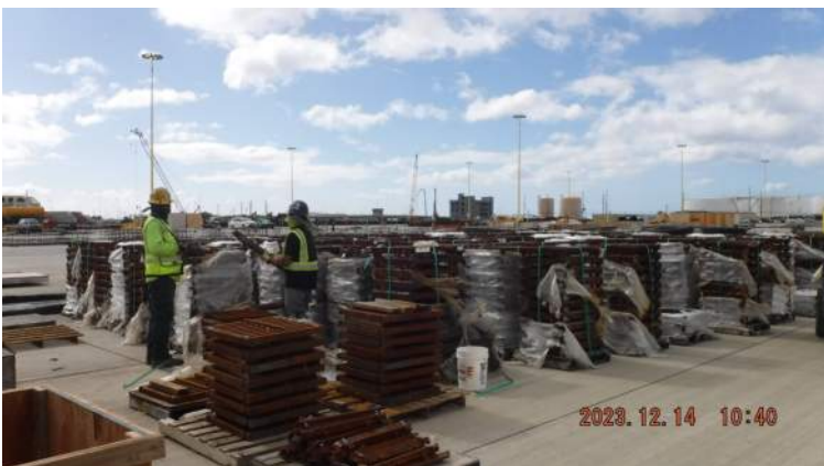
PCCP: KIWC carpentry crew unbolted the grate braces from the original assembly
