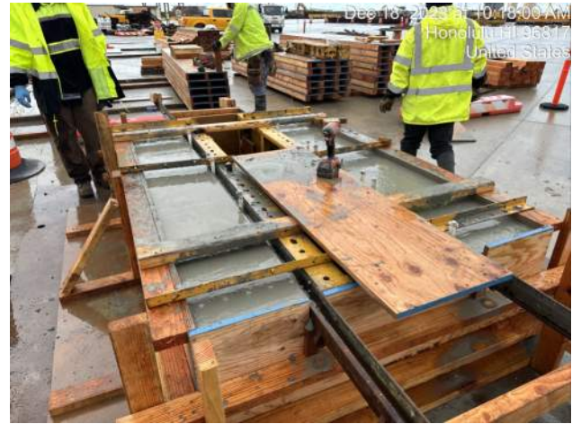
Dec 16, 2023 at 10:18:00 AM Honolulu HI 96817 United States View of the completed mockup pour of TD-3
