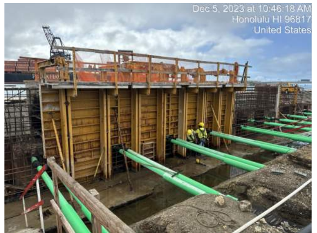
KIWC continued loosening formwork for P7 of the capping beam on Pier 42
