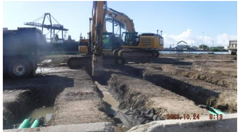
Pier 42: KIWC civil crew (Brent's crew) continued to excavate the subgrade for the installation tie rods between STA 7+00 to STA 7+50
