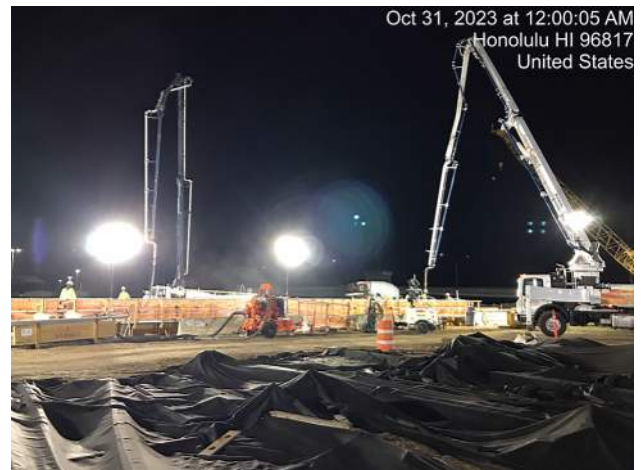
KIWC starting second lift (approximately 40 minute lift timing) for P6 of the LSCRB on Pier 43
