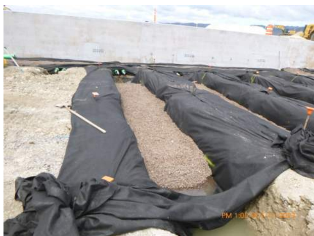
KIWC installing a 1' lift of 3b beneath the tie rod sets in snug harbor.
