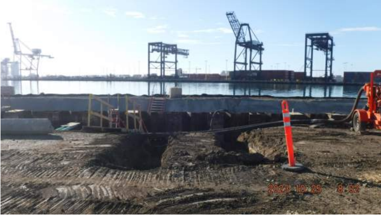
Pier 42: KIWC civil crew continued to excavate the subgrade between STA 12+00 to STA 12+50 for tie rod installation
