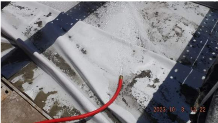
Pier 42: Water was supplied to the top of the concrete pour for curing purposes of Pour #3 of the CWCB
