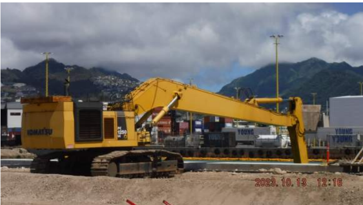
Pier 41: The Komatsu PC 1250 excavator is down. No dredging work from noon to end of shift today
