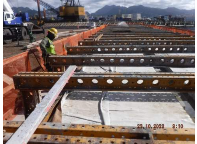
KIWC removing the chamfers from P1 of the LSCRB on Pier 42 to be used on P6 of the LSCRB on Pier 43
