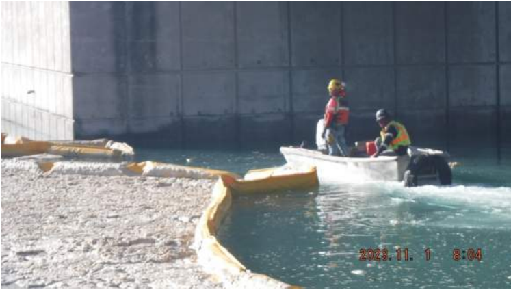
Pier 43: Bridge and Marine crew containing the silt foam within the confines of the silt curtain
