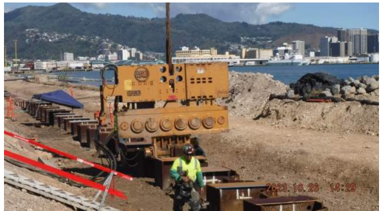
Pier 43: Sheet pile ID # SP422 separated and was re-vibrated to its final tip elevation
