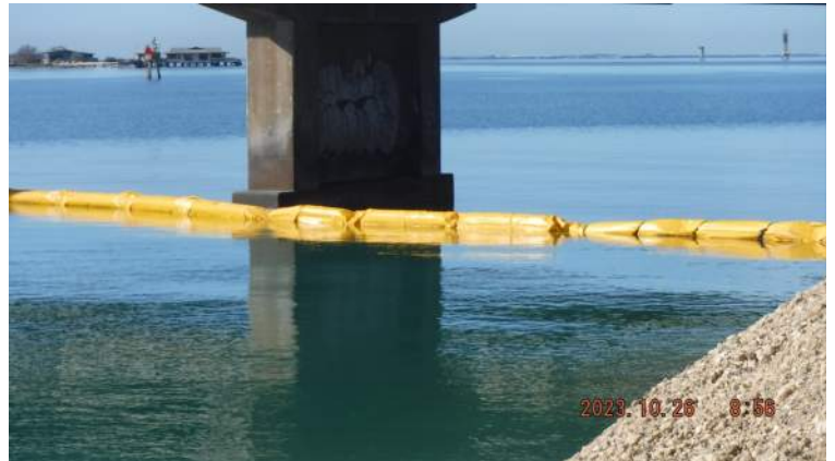
Pier 43: KIWC Bridge and Marine crew continued to fix the silt curtain under the bridge
