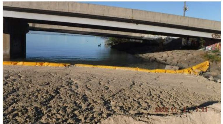
Pier 43: Stone column causeway - View of the silt foam under the bridge within the confines of the silt curtain at 0721 hours
