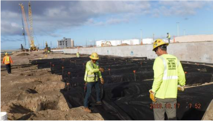
Pier 43: KIWC crew continued to backfill and place #3B fine gravel over the tie rod installation
