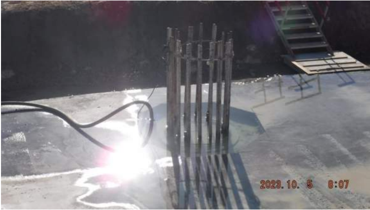
Pier 41: CIDH repair concrete pour at the Deadman extension was cancelled by Micah
