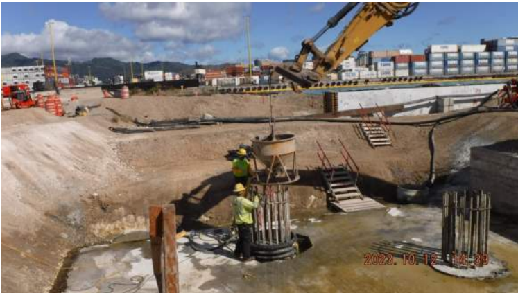
Pier 41: KIWC crew placing concrete mixed over the CIDH repair on the Deadman extension
