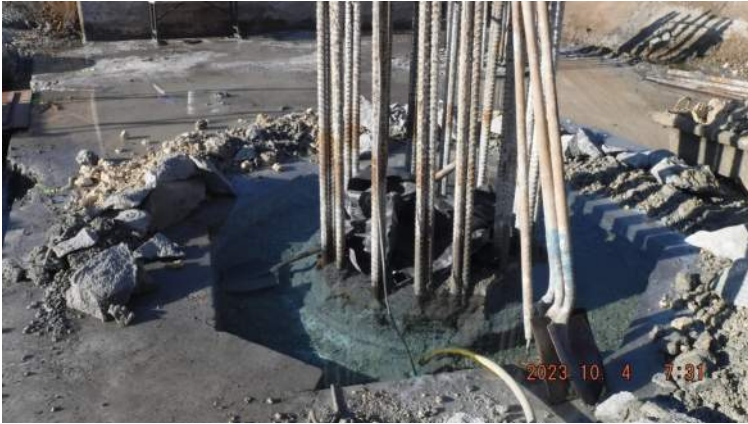
Pier 41: KIWC civil crew continued to chip the mud mat to expose the CIDH pile without concrete cover on the rebars
