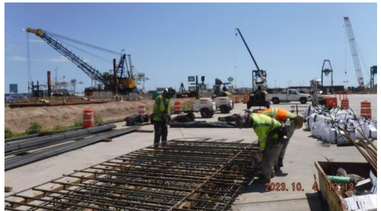
PCCP: Across Pier 41 - HRSPI continued fabricating the rebar cage for the spread footing of ID#3
