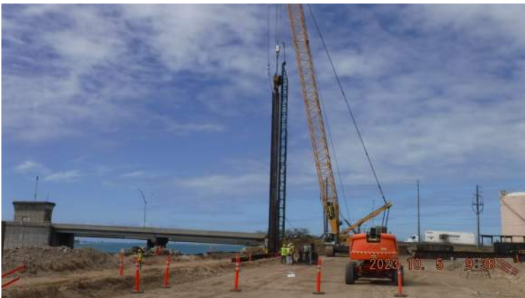
Pier 43: KIWC Bridge and Marine crew continued to drive the king piles
