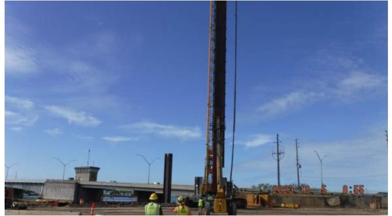
Pier 43: KIWC Bridge and Marine crew continued to drive the king piles
