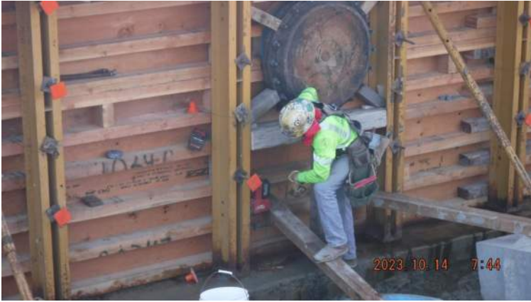
Pier 42: KIWC carpentry crew (Jesse's ) continued to adjust the footing braces for the metal forms of Pour #1 of the LSCRB
