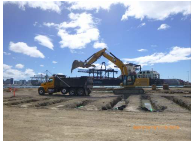
KIWC extending tie rod trenches towards the combi wall along snug harbor.
