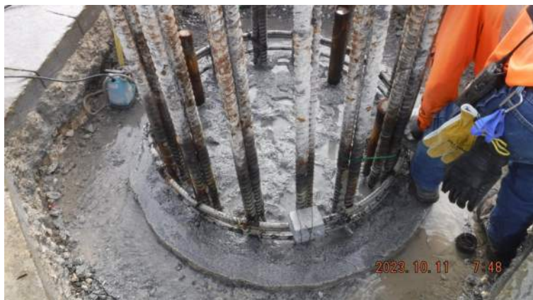
Pier 41: P0 Deadman Extension - KIWC civil crew continued forming the forms surrounding the repair for the CIDH
