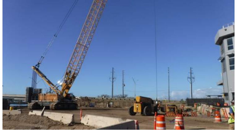
Pier 43; KIWC Bridge and Marine crew continued maintenance of the pile driving equipment
