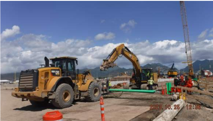
Pier 42: KIWC civil crew continued to install the tie rod assembly from STA 12+00 to STA 12+50
