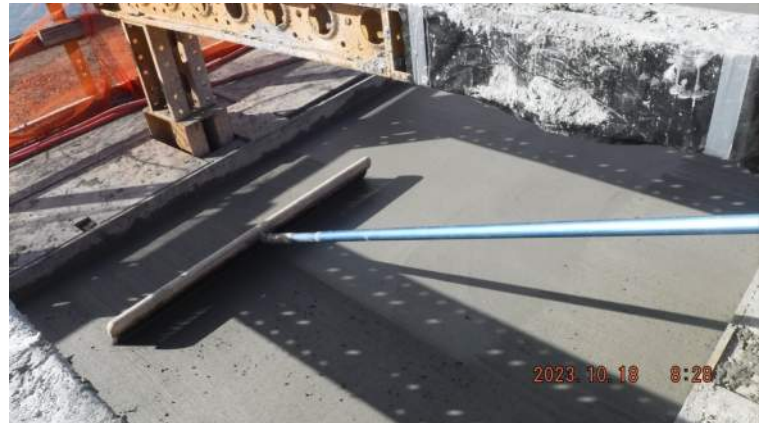
Pier 42: Appearance of the broom finished of the top of the concrete pour for Pour#6 of the CWCB
