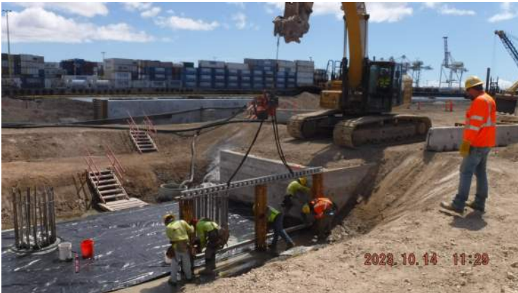
Pier 41: KIWC carpentry crew commenced installing the form template for the P0 Deadman section
