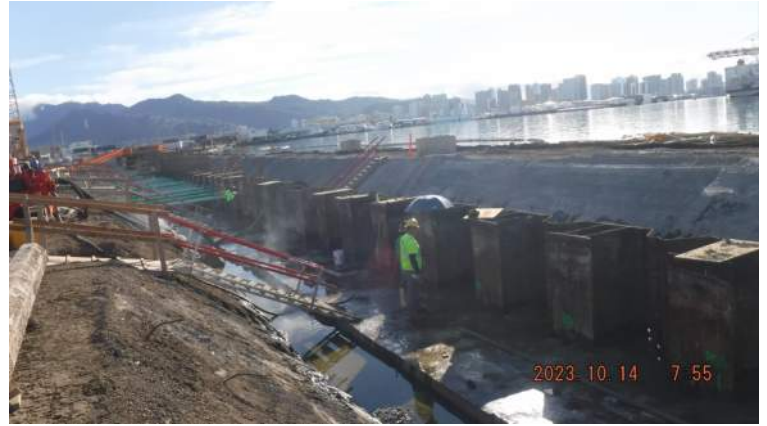
Pier 42: KIWC Bridge and Marine crew continued to lay out and burn holes of the CWCB between STA 12+50 to STA 13+75
