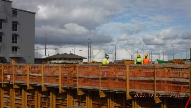
Pier 43: KIWC carpentry crew (Jesses's crew) resumed removing the chamfer and leaned the inside of the rebar cage.
