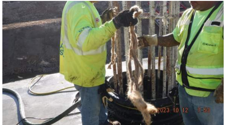
Pier 41: KIWC civil crew ( Micah's crew) used a fiber rope soak into a hydrofoam compound to plug the water from the Deadman extension
