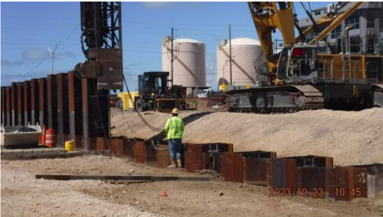
Pier 43: KIWC Bridge and Marine crew continued to drive the double king piles to their final tip elevations
