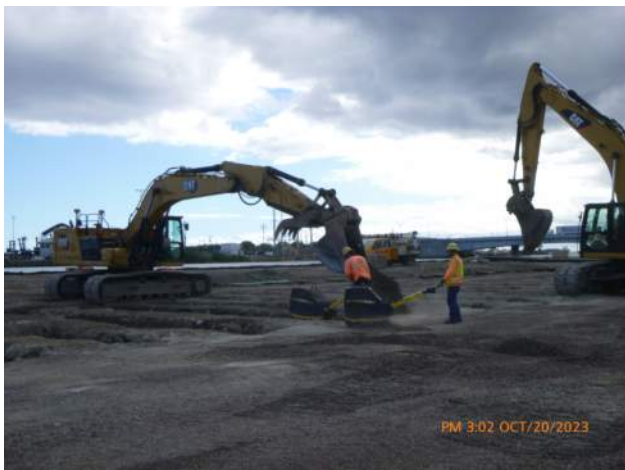
KIWC backfilling over tie rods between the combi wall and the anchor wall.
