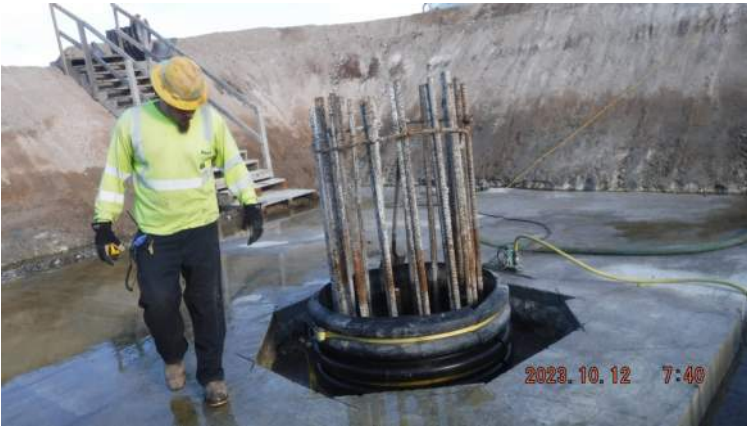
Pier 41: KIWC civil crew ( Sanu's crew) continued dewatering the CIDH repair prior to pouring concrete on PO Deadman extension
