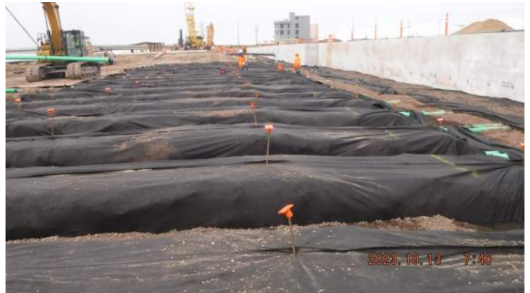
Pier 42: Between STA 6+50 and STA 7+50 - KIWC civil crew (Brent's crew) continued to install the tie rod assembly
