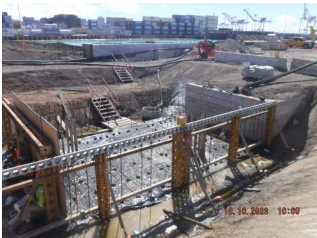
HRSPI progress installing the reinforcement for P0 of the deadman on Pier 41
