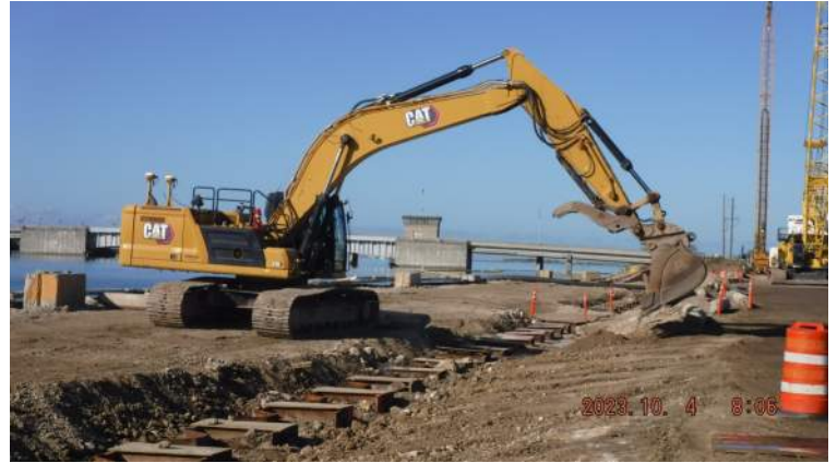
Pier 42: KIWC civil crew continued excavating the subgrade for the mud mat installation between STA 10+00 to STA 11+00
