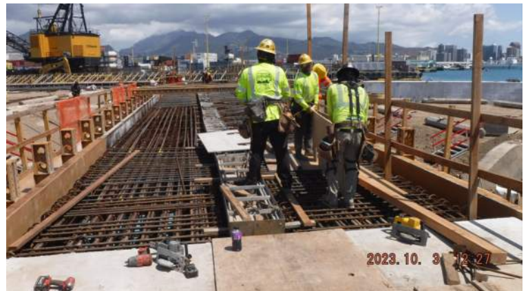
Pier 42: KIWC carpentry crew continued forming the forms for Pour #1 of the LSCRB
