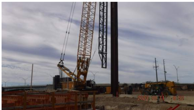
Pier 43: KIWC Bridge and Marine crew continued to drive the king pile by vibratory method
