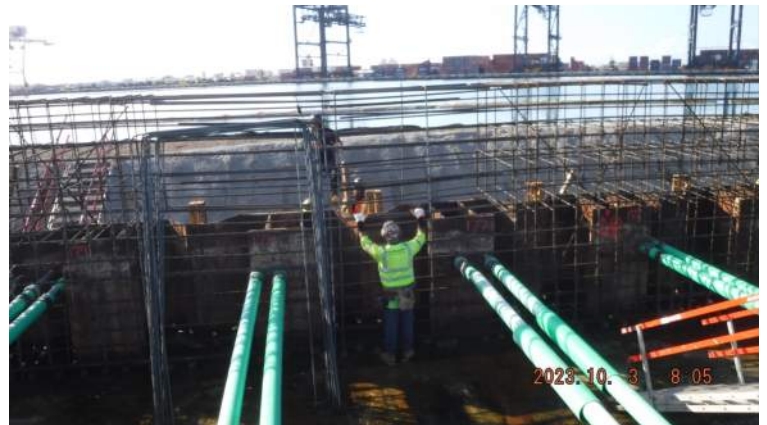
Pier 42: HRSPI crew continued to install the rebar cage for Pour #6 of the CWCB
