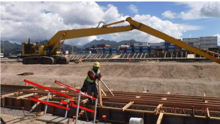
Pier 41: Trench Drain 3 - Carpentry crew forming the sides of the trench drain
