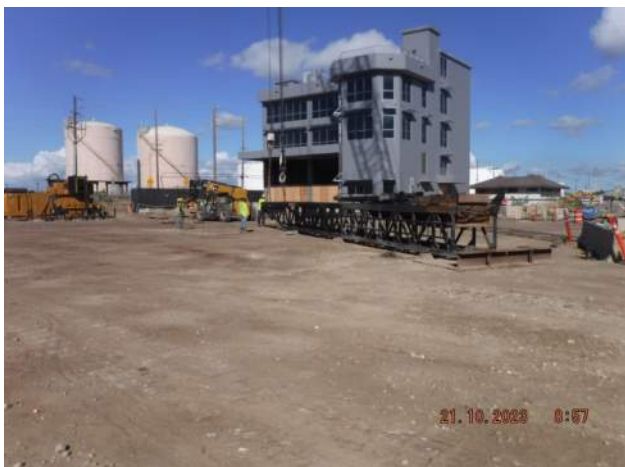
KIWC prepping to use the impact hammer to drive the sheet piles to depth on Pier 43
