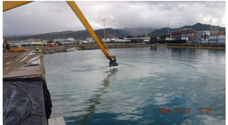
Pier 41: KIWC crew continued to dredge the ocean bottom between Pour# 3 and #4 of the CWCB
