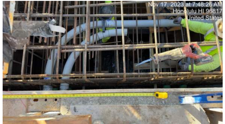
PEC installing two 4" and two 2" conduits in the capping beam P9 on Pier 42
