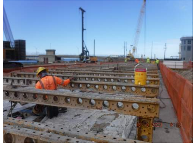
KIWC prepping to remove the crane rail blockout formwork for P5 of the LSCRB
