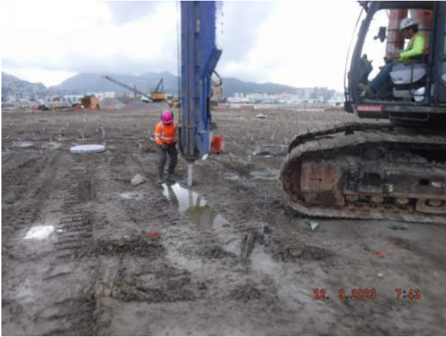
KNA continued installation of wick drains in the Snug Harbor surcharge area
