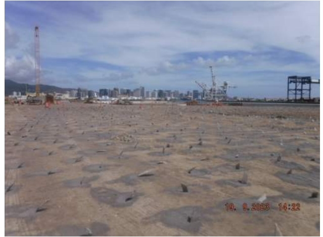
KIWC progress backfilling the wick drains with S4C in the Snug Harbor surcharge area
