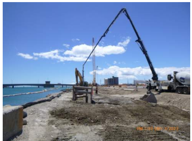
KIWC pouring CLSM for a cut off wall along the waterfront of pier 43.
