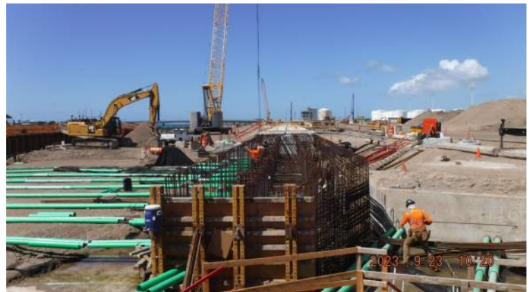
Pier 42: HRSPI crew continued to install the #11 rebar for the walls of Pour #1 of the LSCRB
