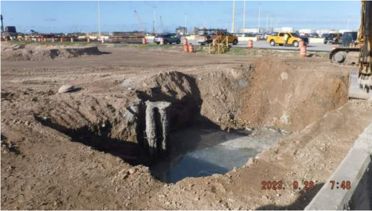
Pier 41: Approximately STA 28+60 to 29+56.6 - KIWC civil crew continued to excavate the subgrade for the Deadman extension
