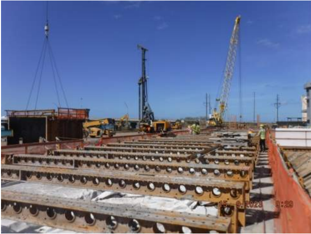
KIWC prepping to fly formwork for installation on P6 of the LSCRB on Pier 43
