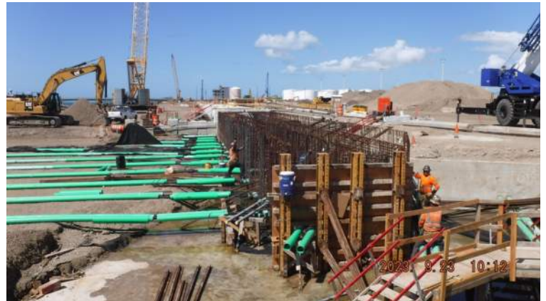
Pier 42: HRSPI crew continued to install the #11 rebar for the walls of Pour #1 of the LSCRB
