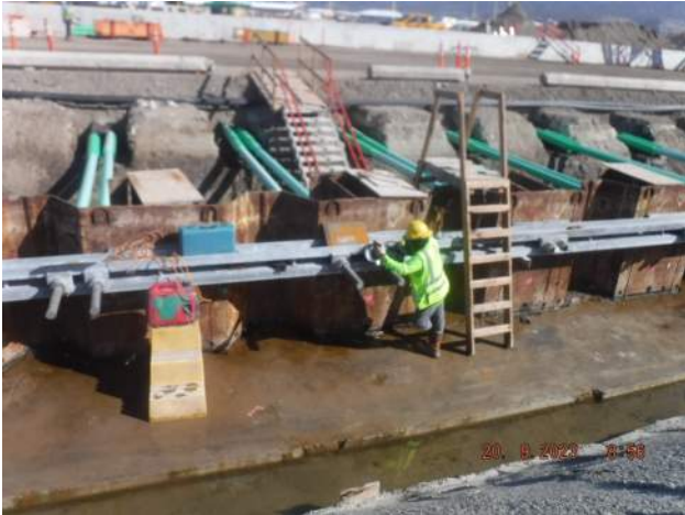
KIWC cutting the ends of the tie rods at the P42 combi wall
