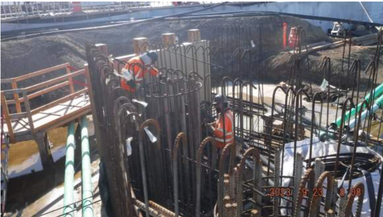
Pier 42: HRSPI crew continued to install the hoops around the CIDH piles
