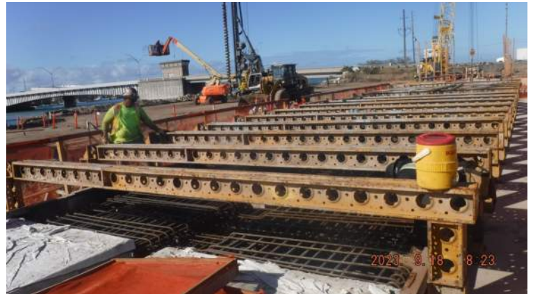
Pier 43: HRSPI crew on site to continue installing the remainder of the stirrups of the top mat rebar cage for Pour #6
