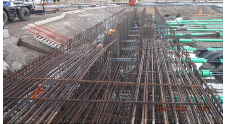
Pier 42: HRSPI crew continued to install the rebar cage for Pour #1 of the LSCRB
