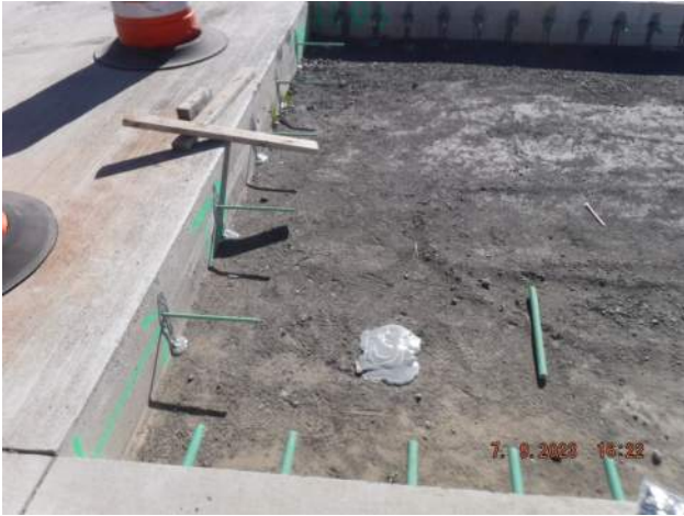
KIWC installed dowels for paving the blockout west of the KIWC construction trailers
