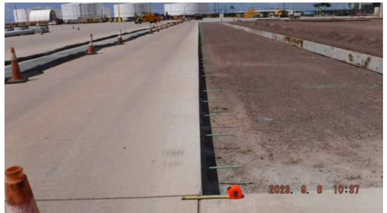
PCCP: Blockout - "A" - East section of the existing PCC not aligned with the expansion seal (15" thick)
