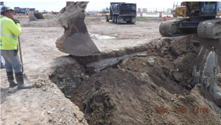
Pier 41: KIWC civil crew continued to excavate the subgrade to expose the north end of the existing Deadman
