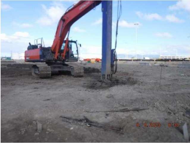
KNA predrilling to 32.5' bgs for installation of wick drains in the Snug Harbor surcharge area
