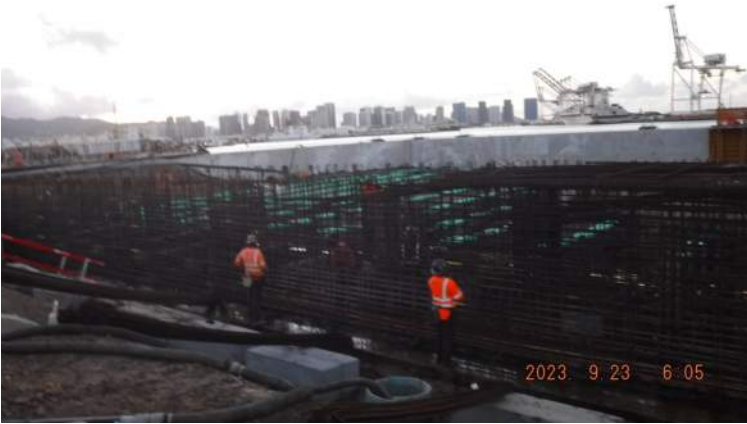
Pier 42: HRSPI crew continued to install the rebar cage for Pour #1 of the LSCRB
