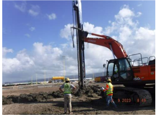
KNA replaced the sheared piece of auger and removed the auger from the ground
