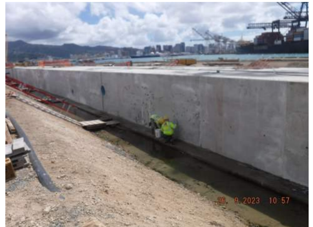
KIWC masons patching the landside of P2 to P4 of the LSCRB on Pier 43
