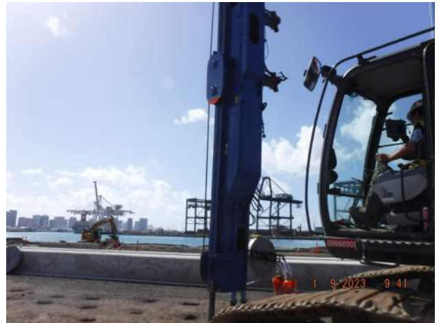
KNA installing a wick drain to 54' bgs due to the GPS system not functioning properly
