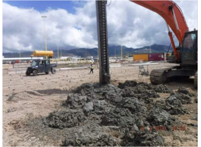
KNA lost 10' of auger 30' bgs in the hole while predrilling for installation of the wick drains
