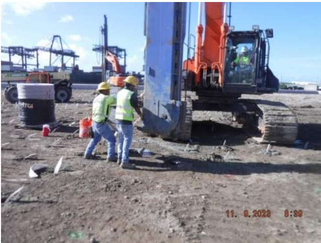
KIWC and KNA installing wick drains in the Snug Harbor surcharge area
