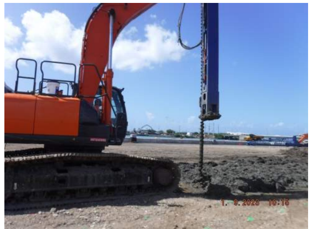
KNA continued predrilling for installation of wick drains while the GPS system is being adjusted for the wick rig
