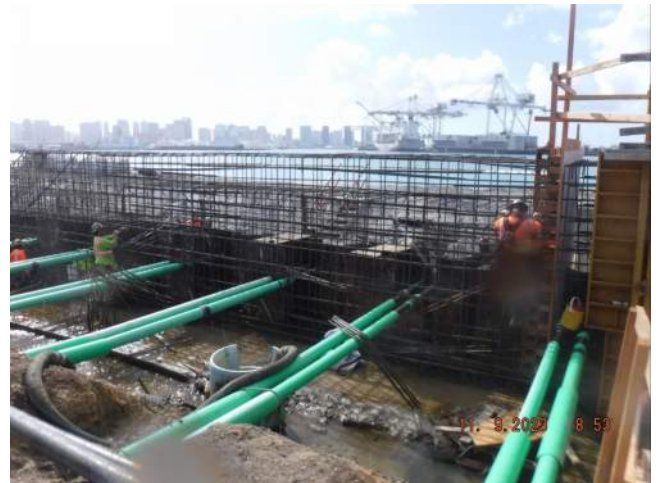
HRSPI installing the reinforcement for P3 of the cap beam on Pier 42
