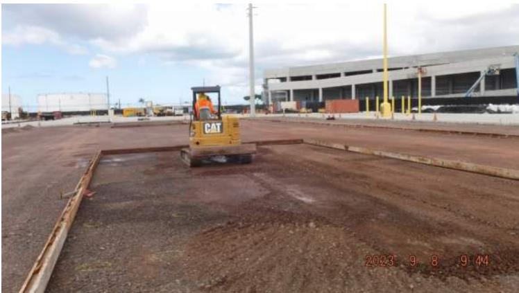
PCCP: Block out "A" - KIWC civil crew used the CAT 304 mini excavator to grade the basecourse aggregate
