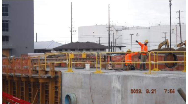
Pier 43: KIWC carpentry crew continued to strip the forms from Pour #5 of the LSCRB
