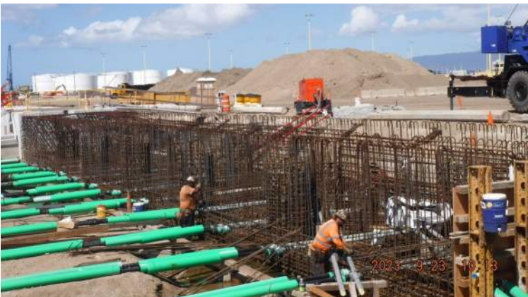
Pier 42: HRSPI crew continued to install the #11 rebar for the walls of Pour #1 of the LSCRB
