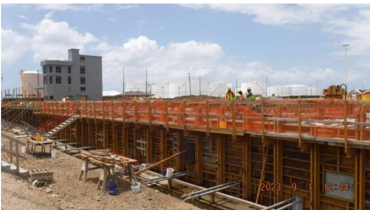
Pier 43: KIWC carpentry crew continued to install the chamfers and adjusted the top cross beams
