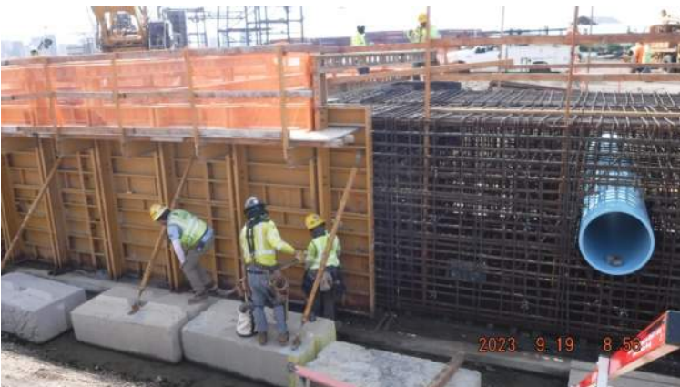
Pier 43: KIWC carpentry crew continued to install the wooden forms for the storm drain on the land side of the LSCRB
