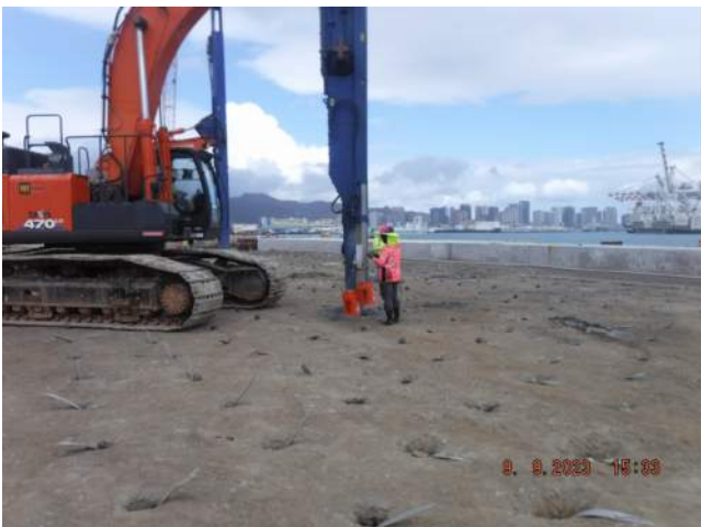
KNA installing wick drains for the remediation areas in the Snug Harbor surcharge area
