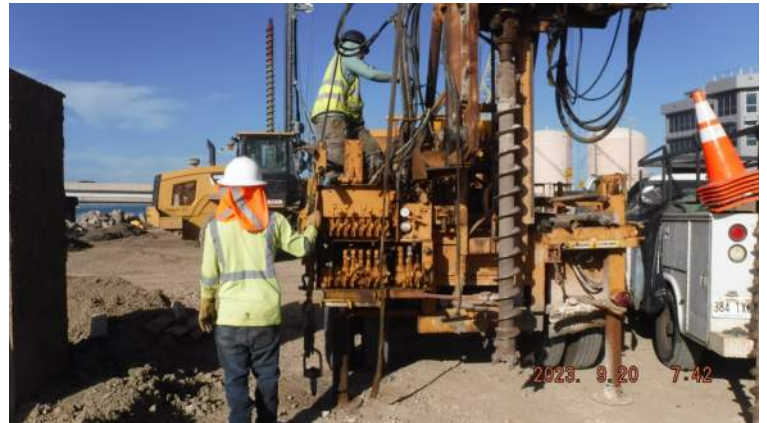
Pier 43: KGI crew set up the drill rig for SPT sampling verification boring # 173
