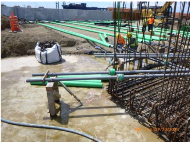
KIWC installed a new 30' tie rod for one of the skewed tie rod sets in LSCRB pour #1.
