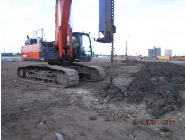
KNA predrilling for installation of wick drains in the Snug Harbor surcharge area
