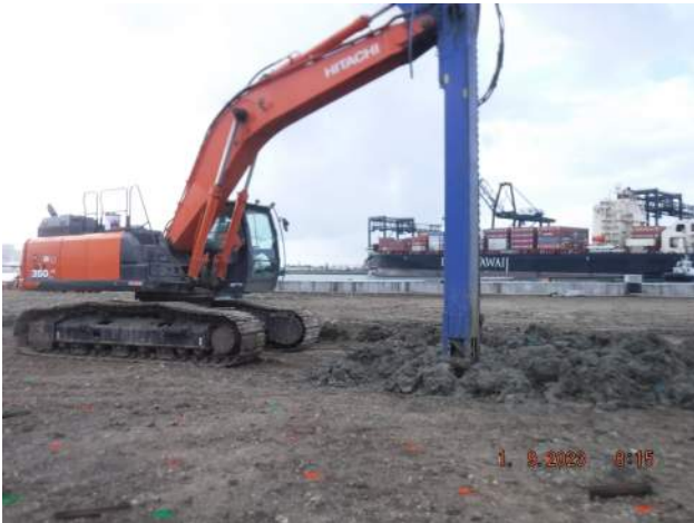
KNA continued predrilling for installation of wick drains at the Snug Harbor surcharge area
